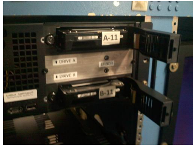
(a) Instrument data system with data drive bay doors open and drives partially removed.
